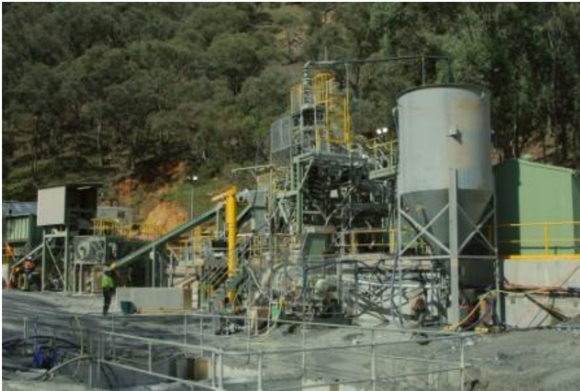
Figure 3:8 Hill End Project – Small Scale Gravity Concentrator Plant
